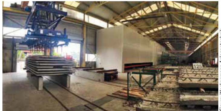
4 x stacker stations for precast floor slabs with 2 x run-off carriages in semi-automatic mode
